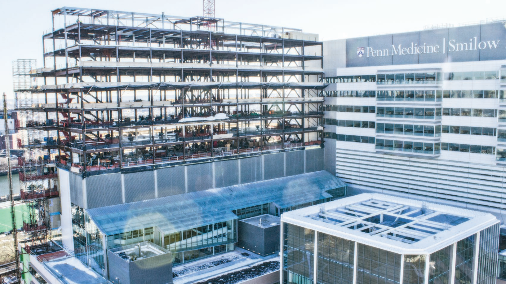
Seen here during construction of the South Pavilion tower of the Perelman Center for Advanced Medicine, the glass-encased Jordan Medical Education Center (with slanted roof and terrace at center) is physically interconnected with the Penn Medicine clinical and research enterprise.
